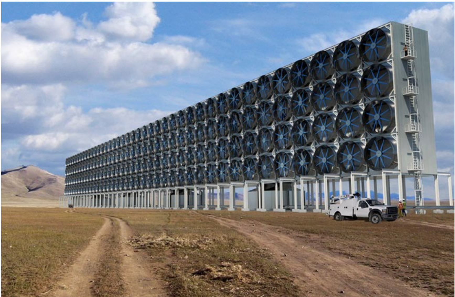
Banks of fans blow air through a CO 2 -capturing solution in this rendering of a direct air capture plant.
